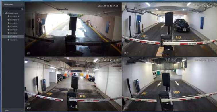
Real time monitoring entrance & exit
